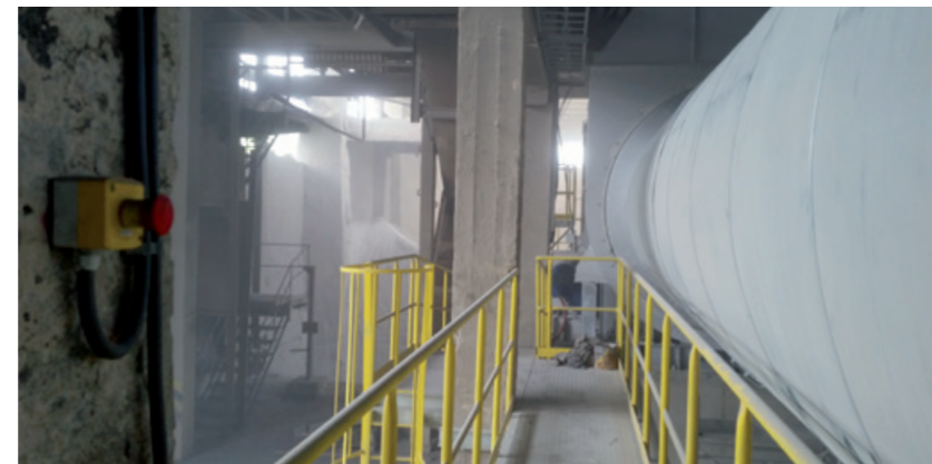
Drying/cooling drum in operation
