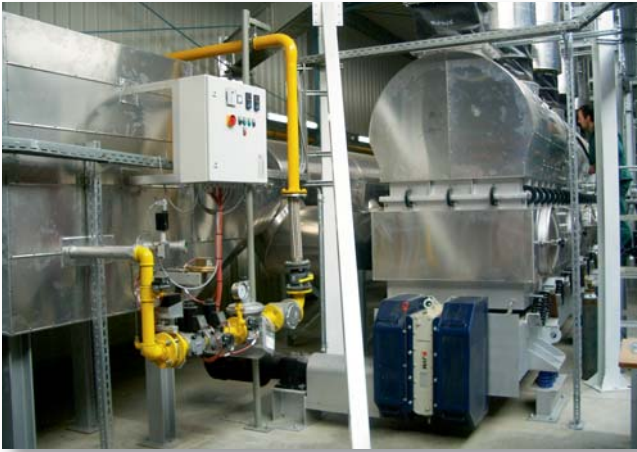
Figure 9: Fluidized-bed dryer for drying recycled plastics with a natural gas surface burner for generating the hot air.
