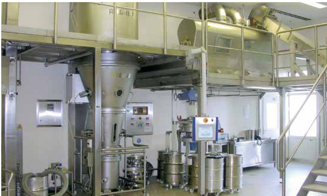
Pharmaceutical drying and coating system
