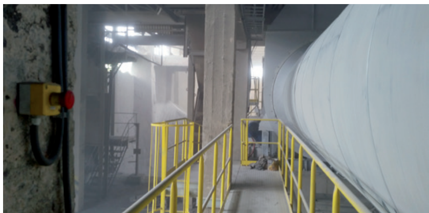
Drying/cooling drum in operation
