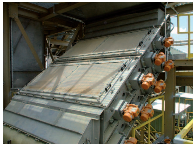
ND 2530 with Plexiglass Hoods – Screening of Wood Chips
