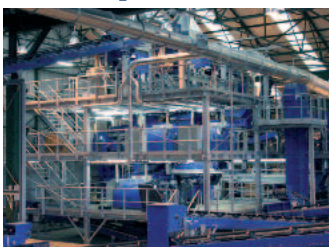
Example: Glass Recycling Plant
