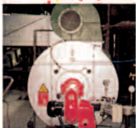
with an intermediate hot gas generator (for sensitive materials)
